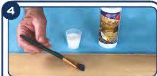
4 Apply an initial coat of Eze-Kote resin and allow it to dry.
