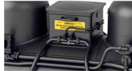
Free-standing pipes on the boiler
